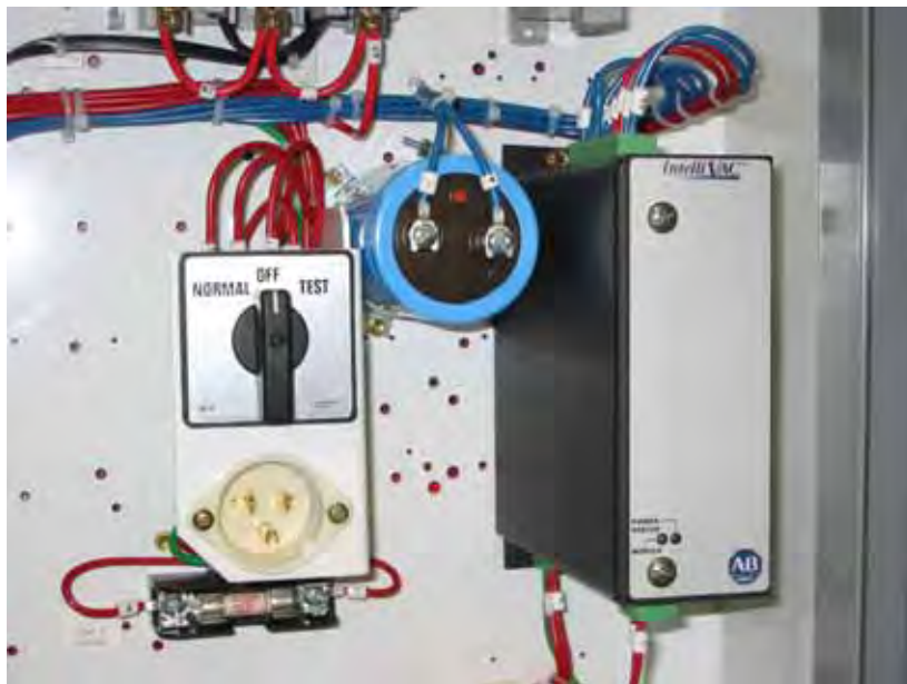
Figure 3.1 - Typical IntelliVAC Installation within a Bulletin 1500/1900 MV Controller (Shown with optional external capacitor)
