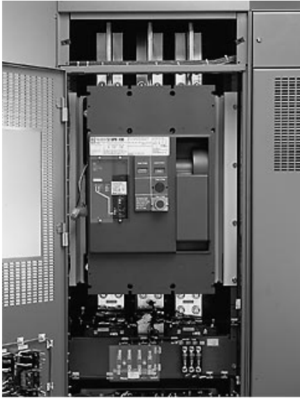
Circuit Breaker in a 3000A DC 1395 Drive
