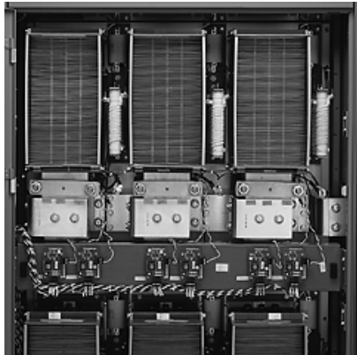
Heatpipe Assemblies in a 3000A DC 1395 Drive
