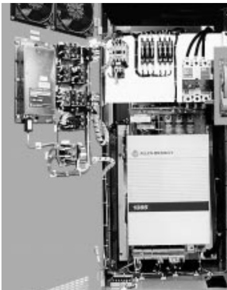
A 110A DC 1395 Drive mounted in an MCC
